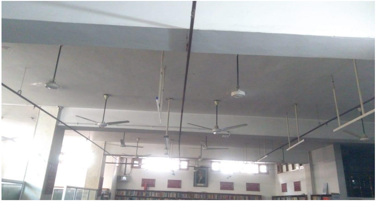
Water Sprinklers for Fire Safety
